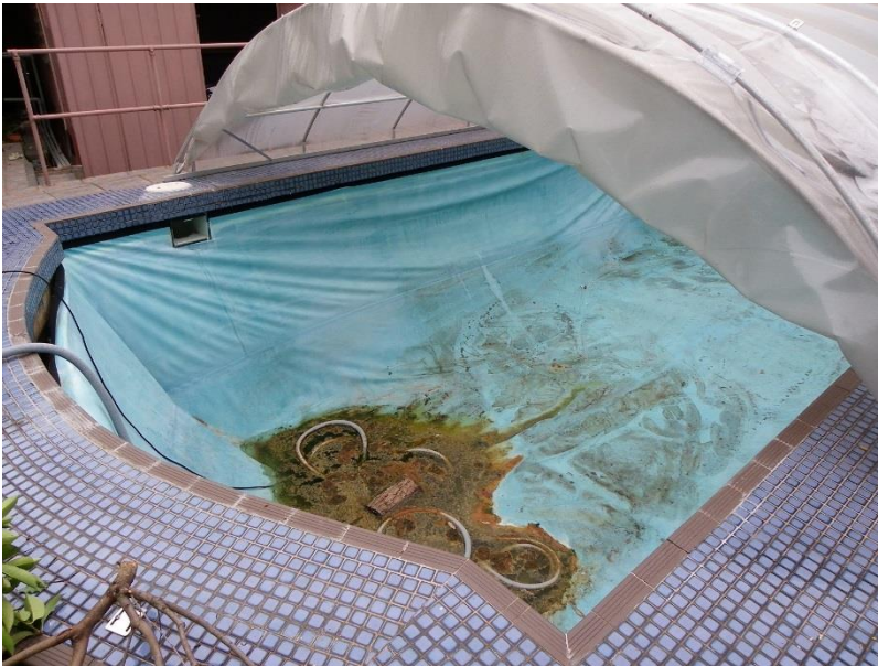
Pic 1. Here the liner has broken away from the fastenings and torn. Also, water has now got behind the liner making it difficult to use and providing an unhealthy water situation.
