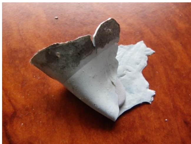
Pic 1. Paint sample showing a “clean” underside indicating insufficient adhesion due to poor surface preparation and also mold present.
