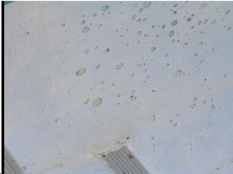
Pic 2, showing blisters (broken) as the result of Hydrostatic pressure.
